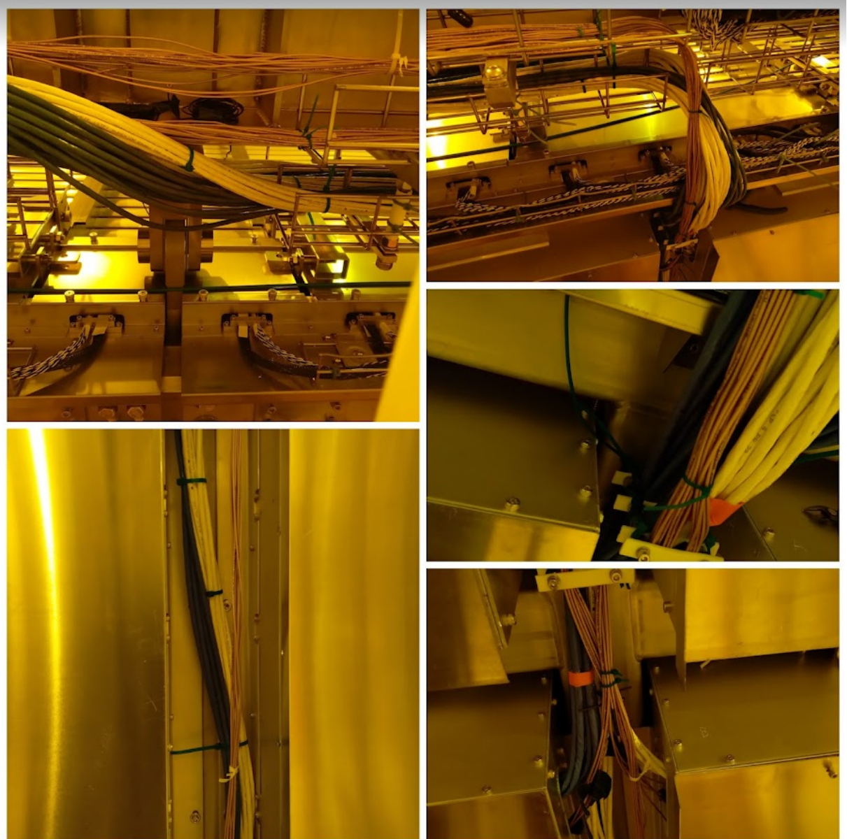
Figure 27 – Views of the PDS cables sitting in tray and routed along the APA
